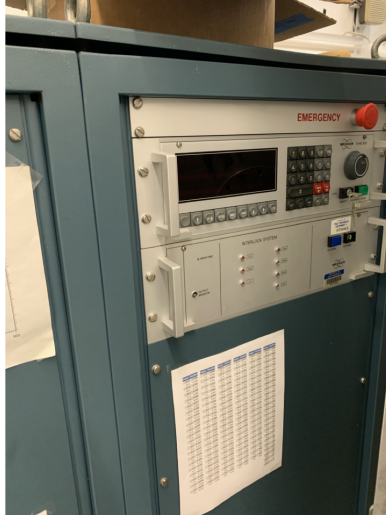
Figure 4: SPS Magnet power supply and control panel
